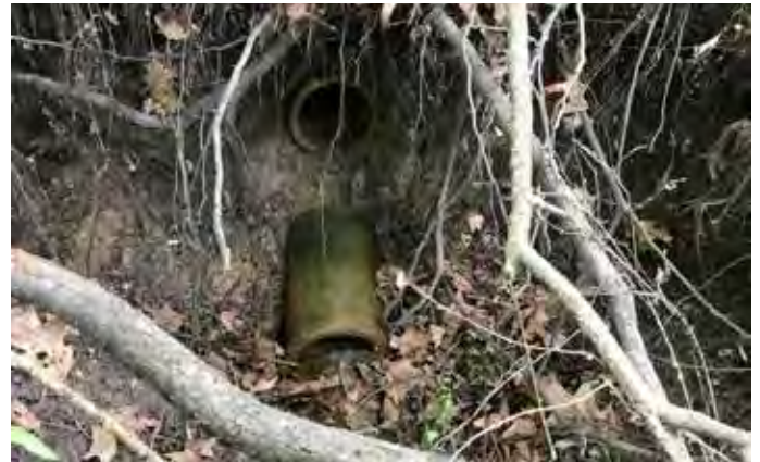
ONE OF MANY OLD DRAIN PIPES FOUND BELOW BLUFF EDGES
