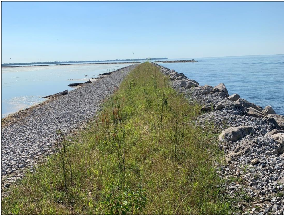
Photo 7. Protective shoals were constructed during restoration to combat erosion along southern end of Celeron Island.
