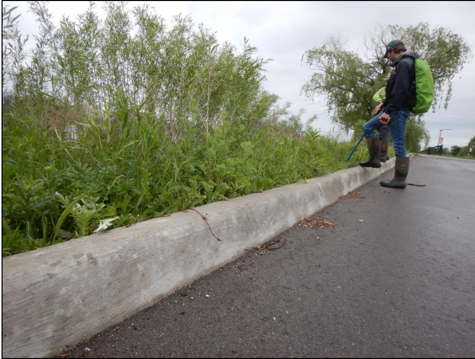
Photo 11. High curb along The Strand Road near the South Fishing Pier on the eastern side of Lake Okonoka.
