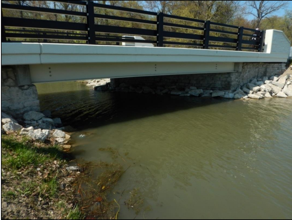
Photo 5. Pre-restoration photo showing the Nashua Canal Bridge with little riprap material and limited snake habitat (HRM 2015).
