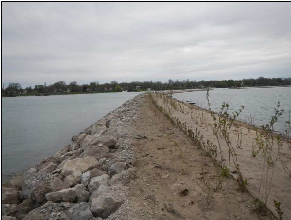
Photo 23. Newly constructed shoal on southern portion of Stony Island including both concrete riprap and planted wetland vegetation.
