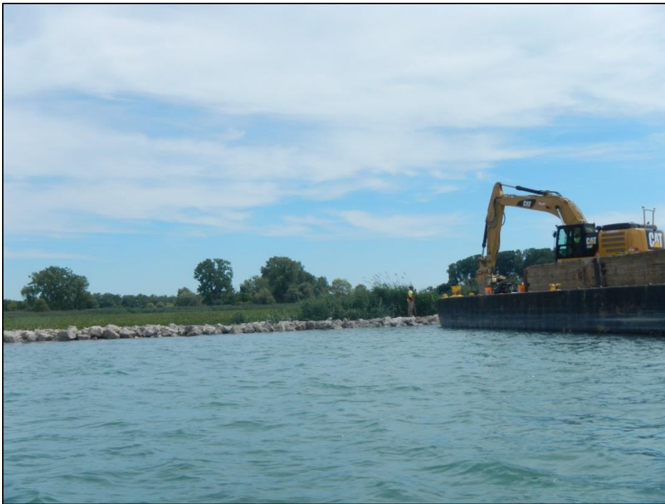
Photo 21. Restoration work underway on the northern portion of Stony Island to construct shoals to reduce further erosion to shorelines caused by heavy wave action.
